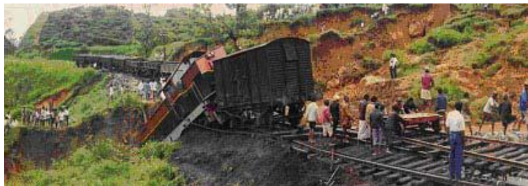
Plate 3: Earthslip at Watanala in 1992. Photo courtesy of National Buildings Research Organization, Colombo, Sri Lanka.
